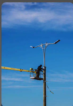
Smart Lamp Pole
